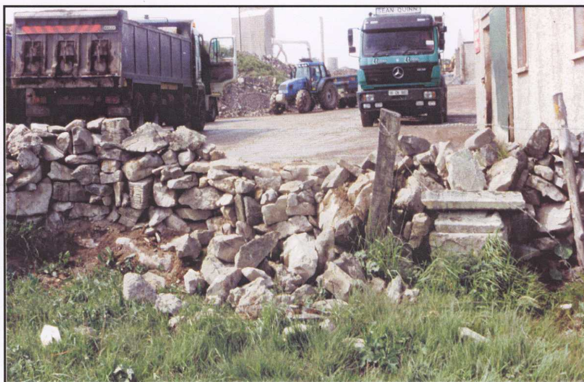
Damaged boundary wall between quarry and Gormans land.
