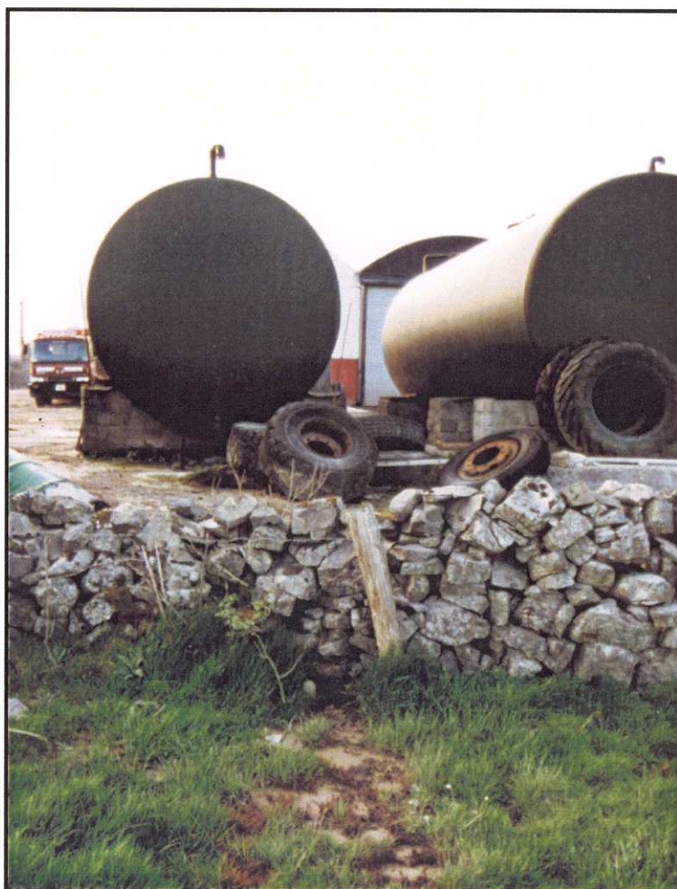
Unbunded storage tanks.
